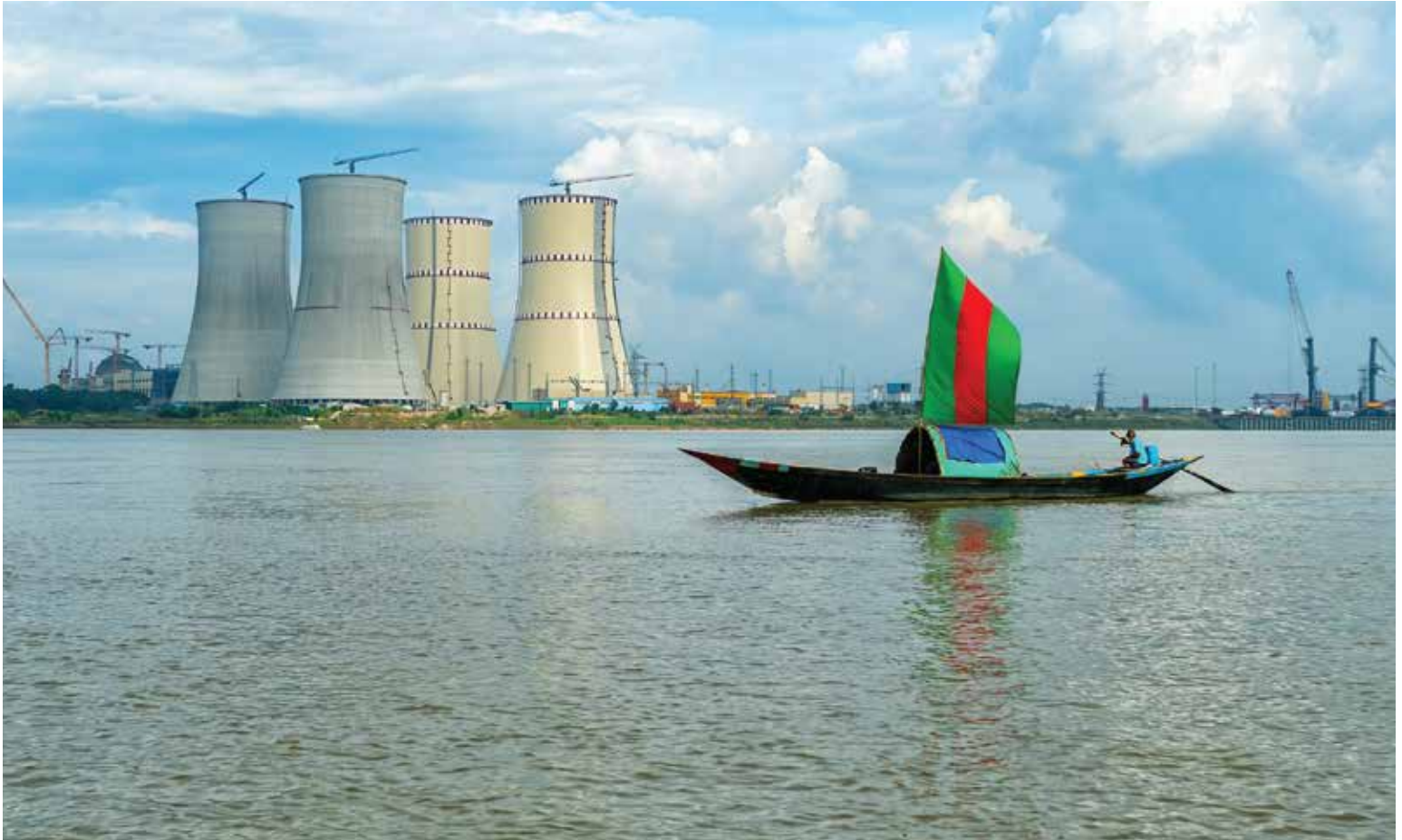
The government of Bangladesh is building its first nuclear power plant in Rooppur on the east side of the river Padma near Ishwardi in the Pabna district of Bangladesh. Photo : Anis Sheikh
